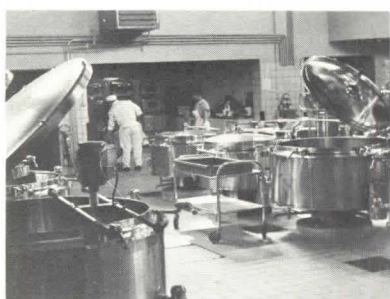
Kitchen, State University Hospital, Ghent
