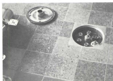
Medical gases outlet, operating theater. Non-explosive gases are used
