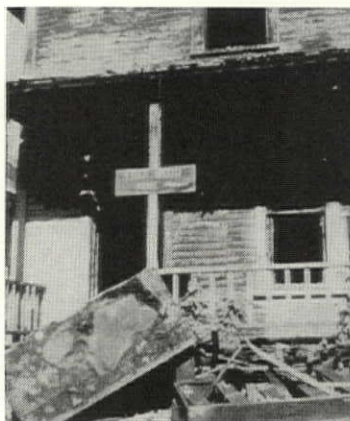
Wood, being indigenous to the area, is seen in abundance as a building material. ALAN CURTIS LIDDLE
