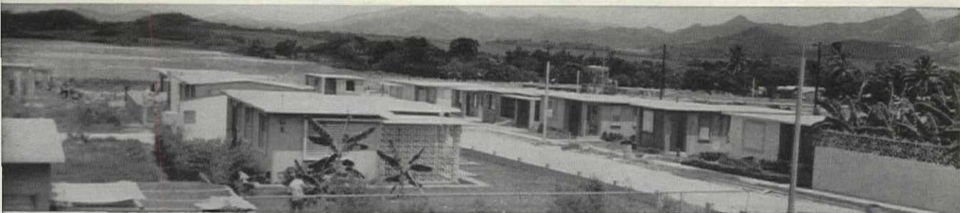
This 34-unit private housing project—known as “La Esperanza”—under construction by contractor Felix A. Torres utilizes “Buckeye” conduit exclusively.
