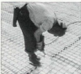
Safe Working Deck is ready the minute Cofar units are welded in place.
