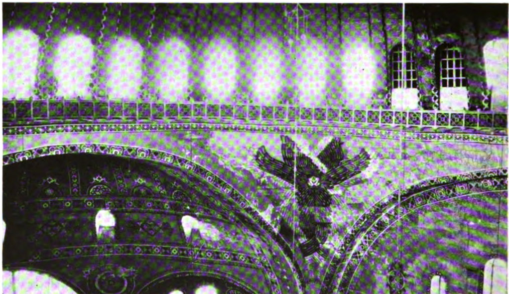
FIGURE 2. THE GALLERY AROUND THE DOME. (Note the distorted arches and the mosaic Cherubim.)
