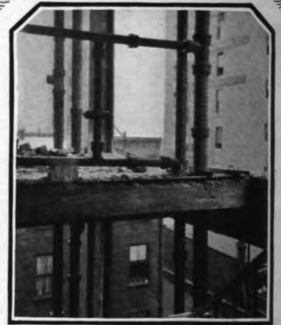
The cast iron soil, waste, vent and leader lines in this 16-Story New York structure will last longer than the building
