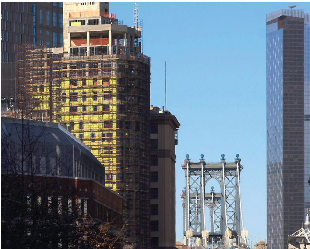
Sealing the building envelope of a Brooklyn high-rise with Georgia-Pacific's DensElement® Barrier System products.
