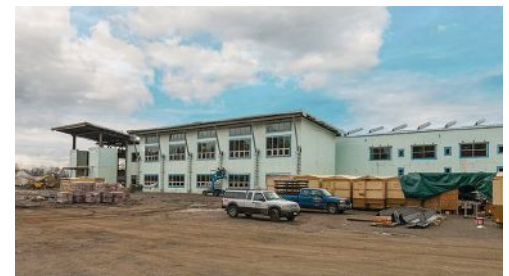
Pierce County Readiness Center Under Construction. Photo: Nudura. See page 1 of this article for completed project.
