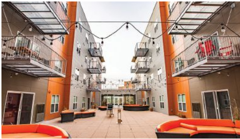
Rainscreens shed most of the rain and manage the rest, preventing moisture intrusion and the resulting premature decay in buildings.
