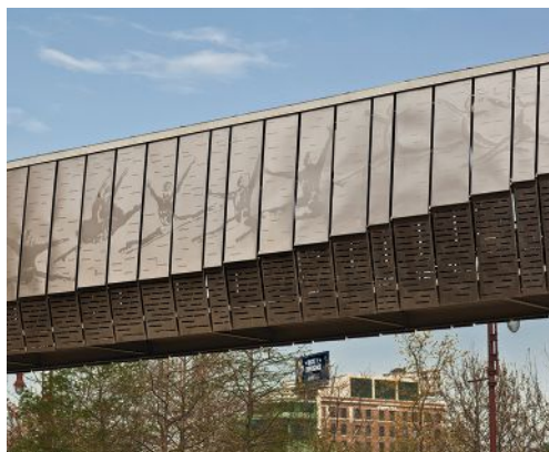
Vector files can be used to create designs in etched and perforated metal—in this case, stainless steel—to make statements of any scale, indoors or out.
