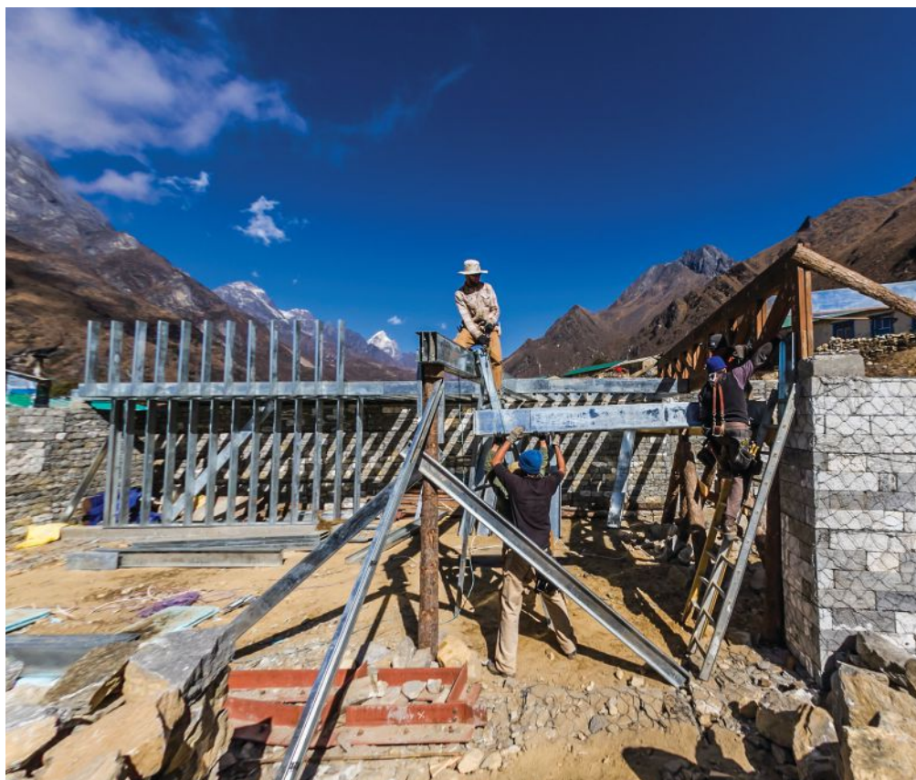
TOP: This traditional puja prayer ceremony is performed before excavation or construction can take place. ABOVE: The crew employs several construction strategies to provide seismic strengthening to the building, including light-gauge steel, stone with gabion cages, and a heavy wood floor truss.
