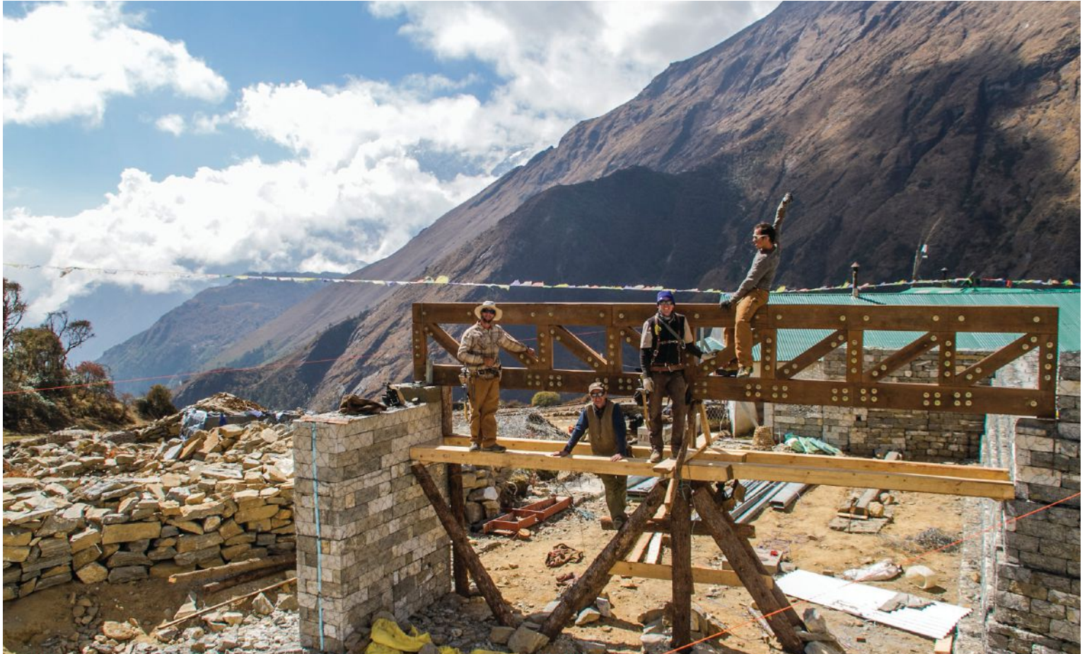
Against a magnificent Himalayan backdrop, a building crew sets the main second-floor truss for the Khumbu Climbing Center.
