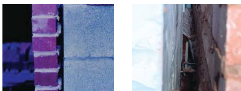
In the photo on the left, the air space is about ¾" inch, and the mortar is almost bridging the cavity allowing water to get deeper into the wall system. In the photo on the right, you can see a larger air space where it would be difficult to create bridges in that air space.
