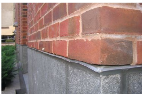
Drip edges are commonly used with flashing to help force the water away from the wall, but designers may not like the appearance of a drip edge in their design.
