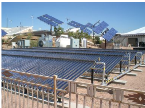
Solar air conditioning uses solar radiation to heat water to drive thermally activated cooling systems. Photo credit: U.S. Army Environmental
