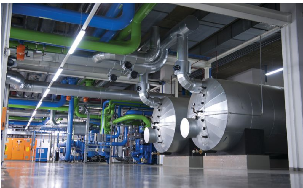
A combined heat and power plant: the gas engine drives a generator to produce electricity while the waste heat is used to warm and cool the building. Photo credit: Bilfinger
