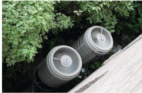
A heat pump can be reversed to either heat or cool a space.
