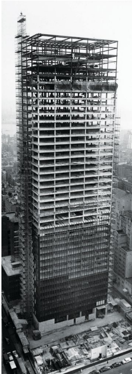
In December 1956, construction on the Seagram was about halfway done, with 38 floors framed out, glass inserted on the seventh floor, and bronze mullions attached up to the 14th floor.
