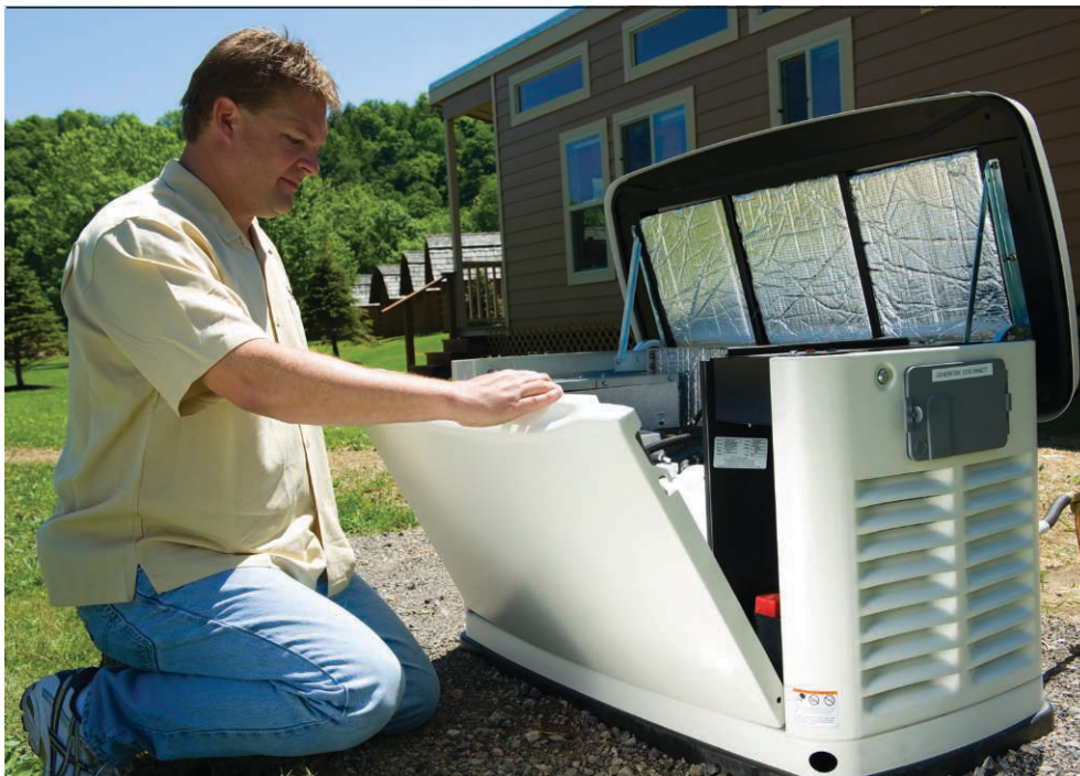
The Herkimer solar-powered lodge's heating system, refrigerator, and domestic hot water system all run off propane, as does the generator. During peak demand the lodge uses about 16 amps, the equivalent of two toasters.
