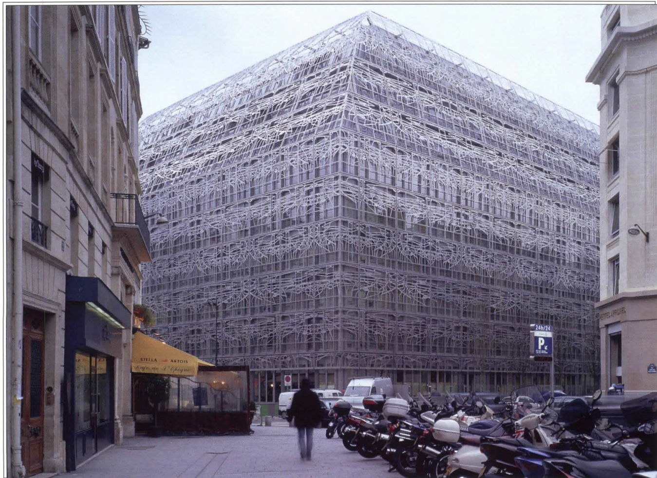
Hundreds of panels of laser-cut, 1/2-inch-thick stainless-steel lattice envelopes the entire façade of the French Ministry of Culture and Communication in Paris. Each panel measures 10 feet by 12-1/2 feet.
