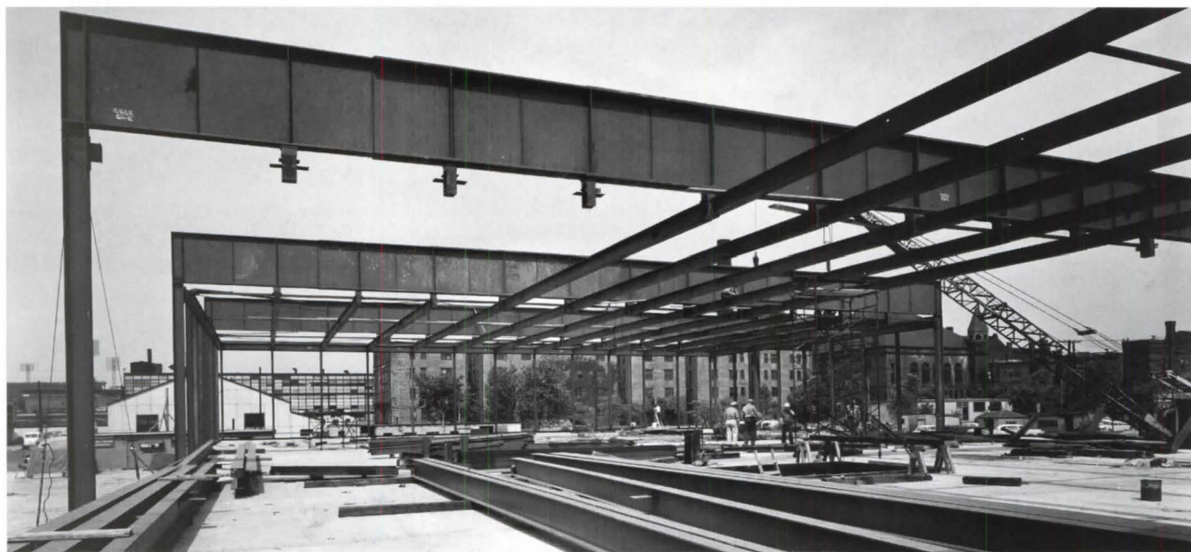
The restoration has not disturbed Crown Hall's four 6-foot-deep steel girders—seen in this archival photograph.
