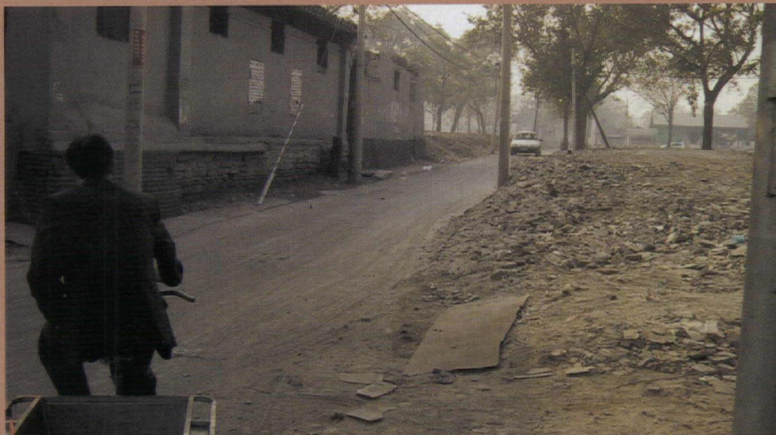
The demolition of this historic hutong in the center of Beijing is typical of the city's wholesale redevelopment.
