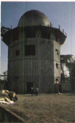
Rusty steel structure (above) contained powerful radar for U.S. military. During renovation, contractor carefully removed lead-based paint and installed windows (facing page, left). Near completion, contractor painted tower painted bright yellow and aquamarine (facing page, right), recalling colors of toucan.
