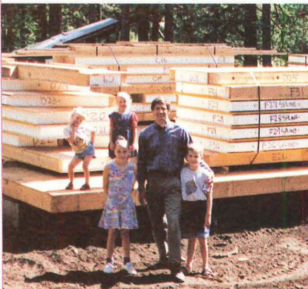
Bear Valley, California, architect David Wright (shown here with his four children) received delivery of SIP panels at 8 a.m.
