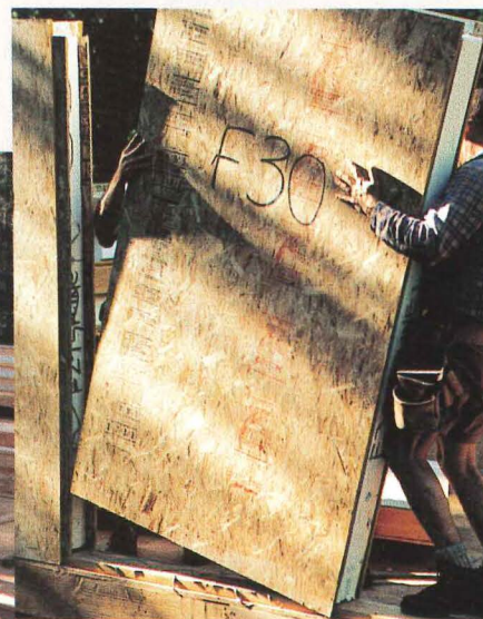
Double-spline joint and bottom plate anchor standard 4'x8' SIP panel into place.
