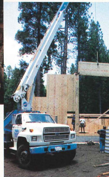
At noon, crane arrives to assist crew in placing large or high panels.
