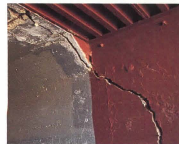
WALLS: Cracks between old and new.
