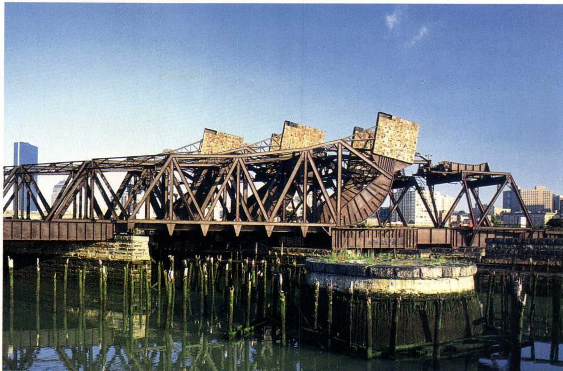
OLD COLONY BRIDGE: Counterweights and rocker arms (right) raise bridge span (left) over channel.
