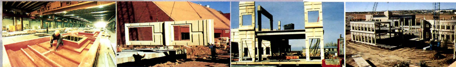
Construction of SOM's Aurora Justice Center illustrates how a mold for a precast element is constructed (inset, far left) and how formwork influences a panel's shape. Transportation and erection of a panel (inset, second from left to far right), also determine the articulation of an exterior.
