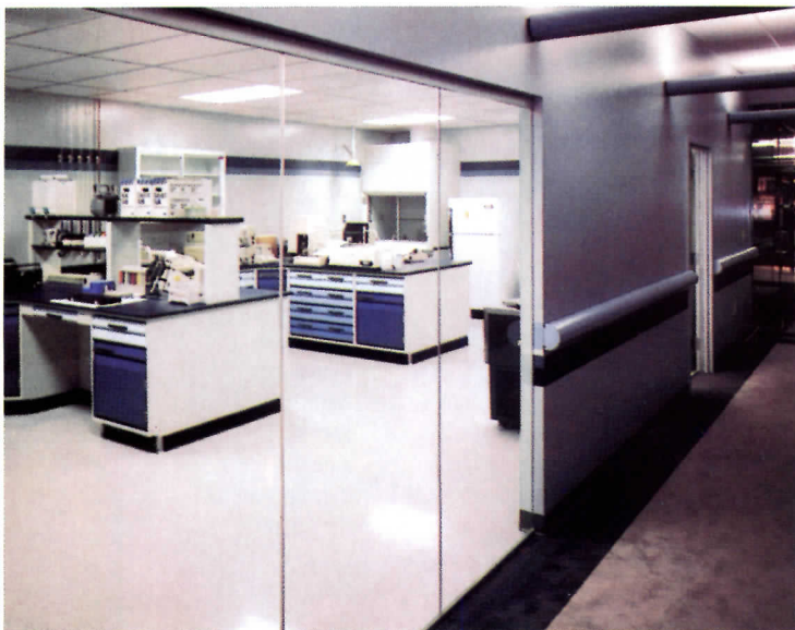
Below, flexible HVAC system of the Serono DNA lab allows a wide variety of lab types. Note observation corridor.
