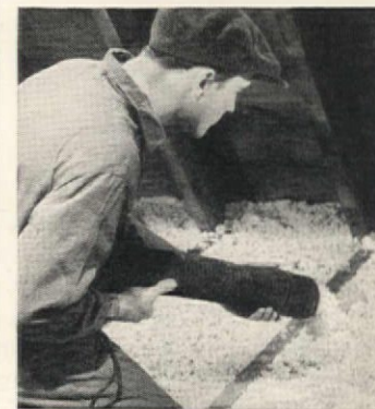
Blowing "rock wool" between attic joists. The empty spaces in the walls can also be filled easily by this method—blanketing the entire house.
