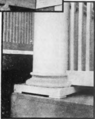
Small openings should be provided in the bases of wooden columns to permit continual ventilation so that the wood will not remain damp for a long period after rain storms and eventually rot at the base. The top photograph shows a typical example of what happens when this ventilation is not provided. Cast iron bases are also successfully used to prevent rotting
