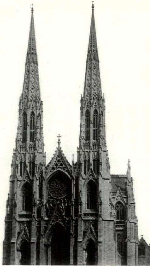
St. Patrick's Cathedral restoration. George A. Fuller Company, New York, N. Y., General Contractors. Maginnis and Walsh, Boston, Mass., Architects.
