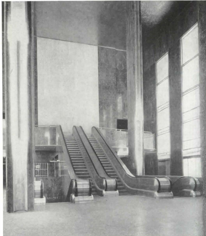
Not the first, but certainly one of the most striking installations of moving stairways in an office building is this one in the lobby of the International Building, Rockefeller Center. Where access to the basement is important, as in this instance, moving stairways make elevator service unnecessary, greatly simplifying operation. Escalators by Otis Elevator Co.
