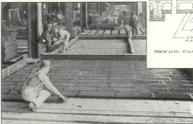
Workmen installing 172,000 board feet of Armstrong's Corkboard over the track level of the Merchandise Mart. Cork serves throughout the building.
