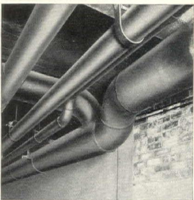
3", 10" and 14" Tube-Turns greatly simplified the pipe-design of this Chase Copper & Brass Company Plant job at Cleveland. The Austin Co., Engineers and Contractors. The Smith & Oby Co., Piping Contractors.
