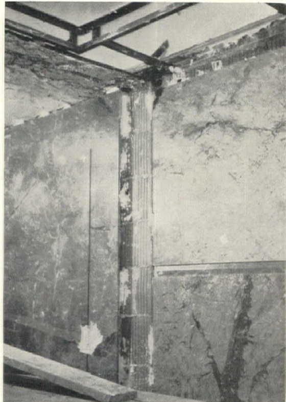
Rose Formosa marble panels and Estrellante trim showing junction of ceiling and light trough
