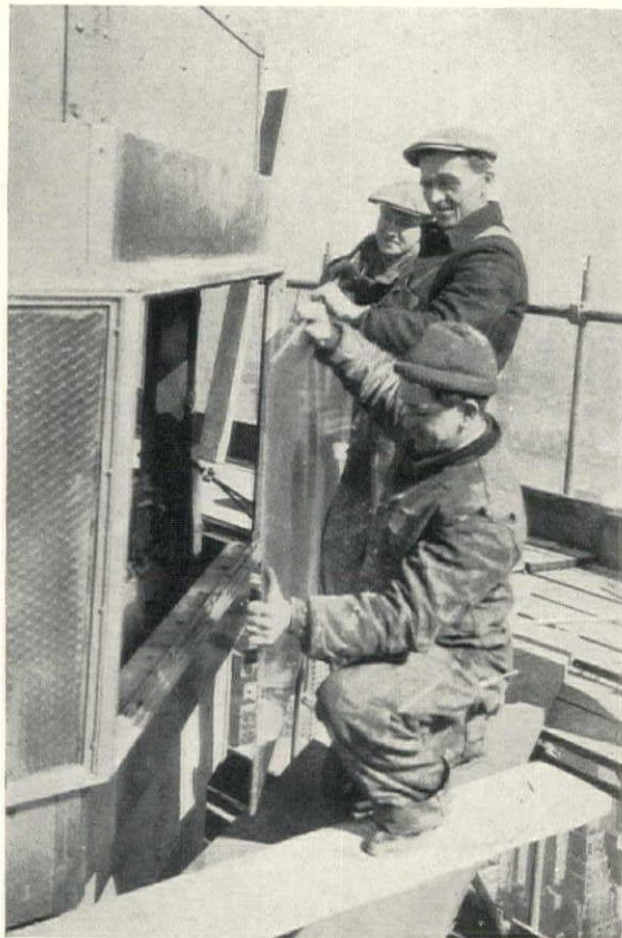
The horizontal ribbed wire glass panels being installed in the section directly below the wings
