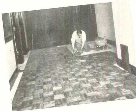
Laying *CELLized oak floor blocks in EVERBOND over a wood subfloor, in a Chicago office building.
