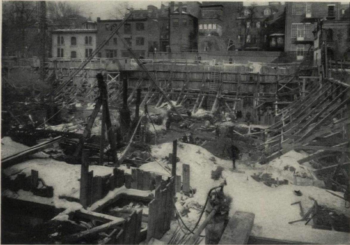
Laborers "Mopping Up" an Overnight Snow Before the Day's Work Starts. Lines of Steam and Shovel and Broom Soon Clear Away an Otherwise Unworkable Area
