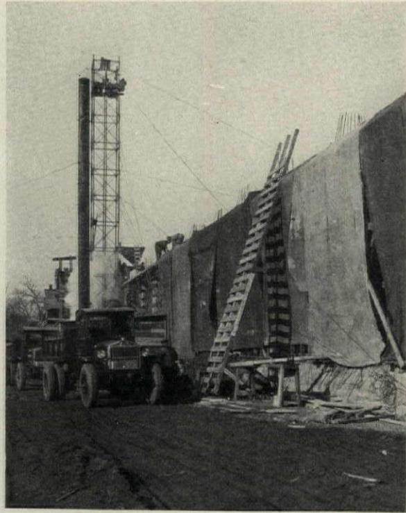
Tarpaulin Coverage for Openings and for Freshly Poured Concrete Wall and Floor Forms is Essential Until the "Set of the Mix" Has Passed all Danger from Freezing Temperatures
