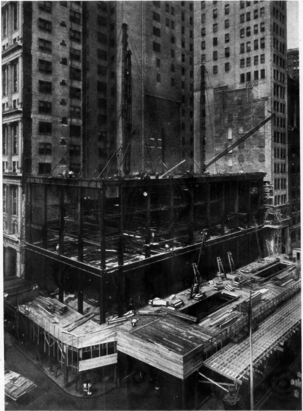
View During Construction, While Cantilever Trusses Were Being Inserted to Support 24-Story Load Originally Carried by Columns in Old Building
