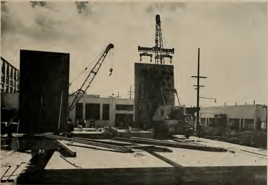
BELOW —two of the huge concrete slab panels have been raised into wall position.
