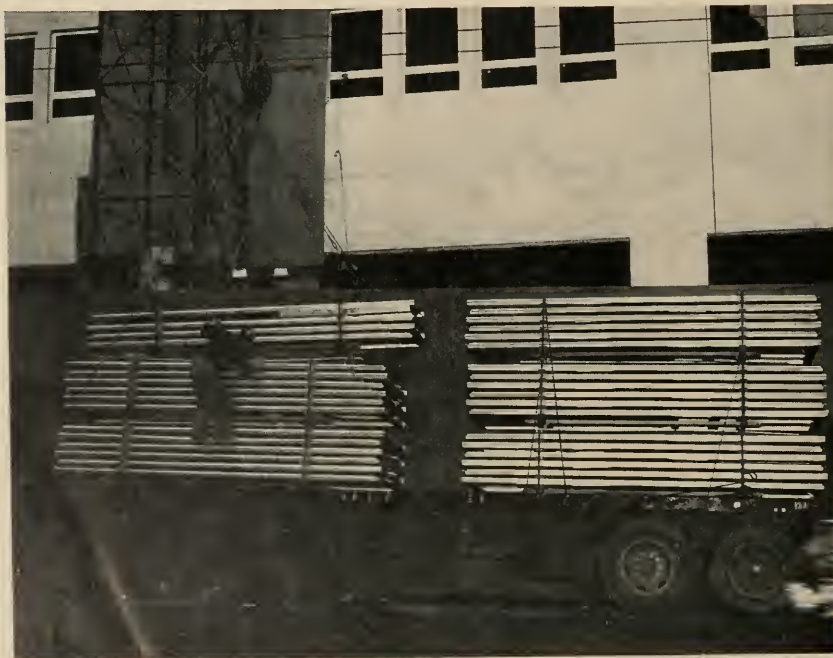
Factory prefabricated frames delivered to jobs on pallets bundled six to each pallet and hoisted to floors.
