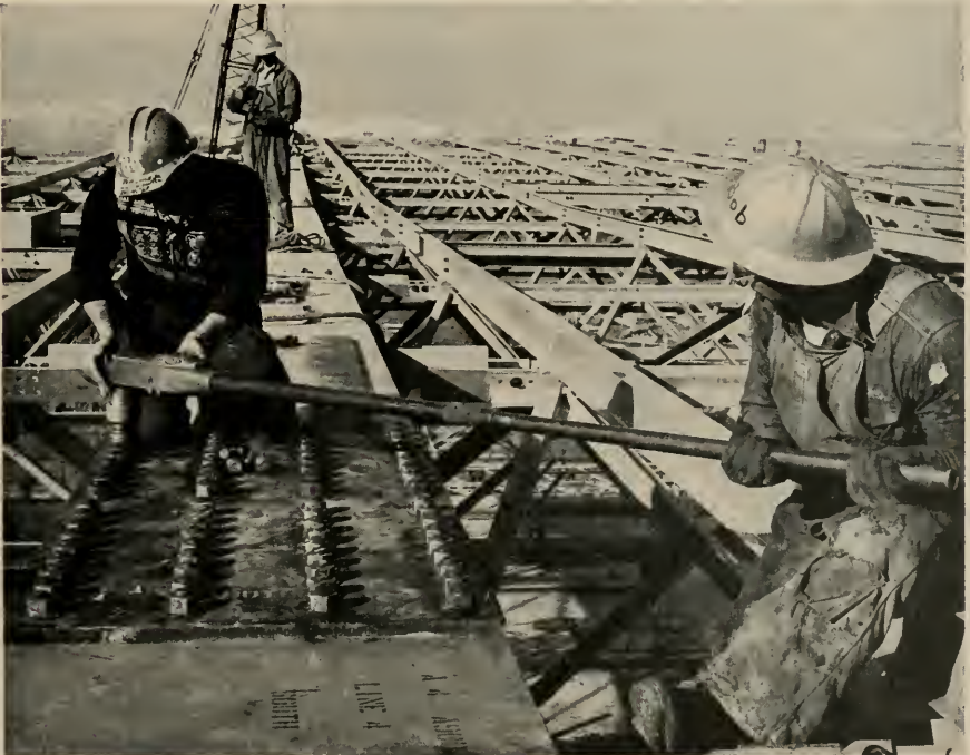
TESTING CALIBRATIONS on high tensile bolts used to splice flanges of 365-ft. girders which cantilever 142-ft. each way.
