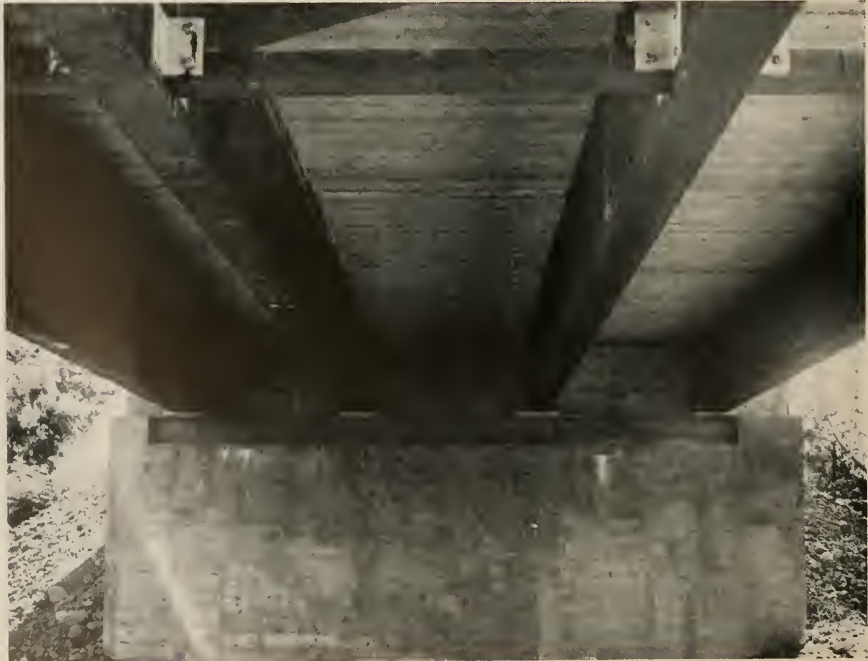
GIRDERS rest upon heavily galvanized steel pads. Diaphragm bracing is located at center of the bridge.
