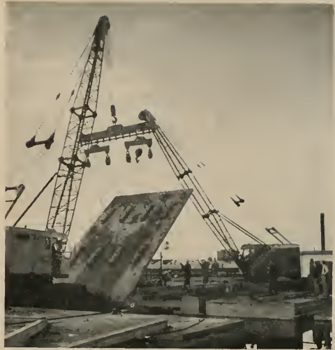
ABOVE —one of the thirty-four panels being raised into final construction position.
