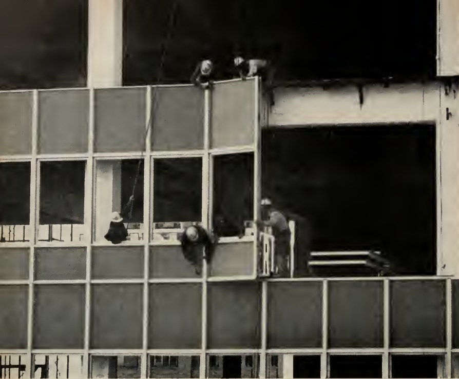
INSIDE SETTING No scaffolding installed in installation of this wall. Note interior back-up pan primed at factory, ready for finish.
