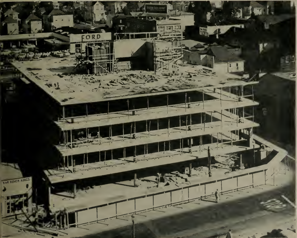
TIOGA BUILDING with floor slabs in permanent position ready far installation of exterior glass walls.
