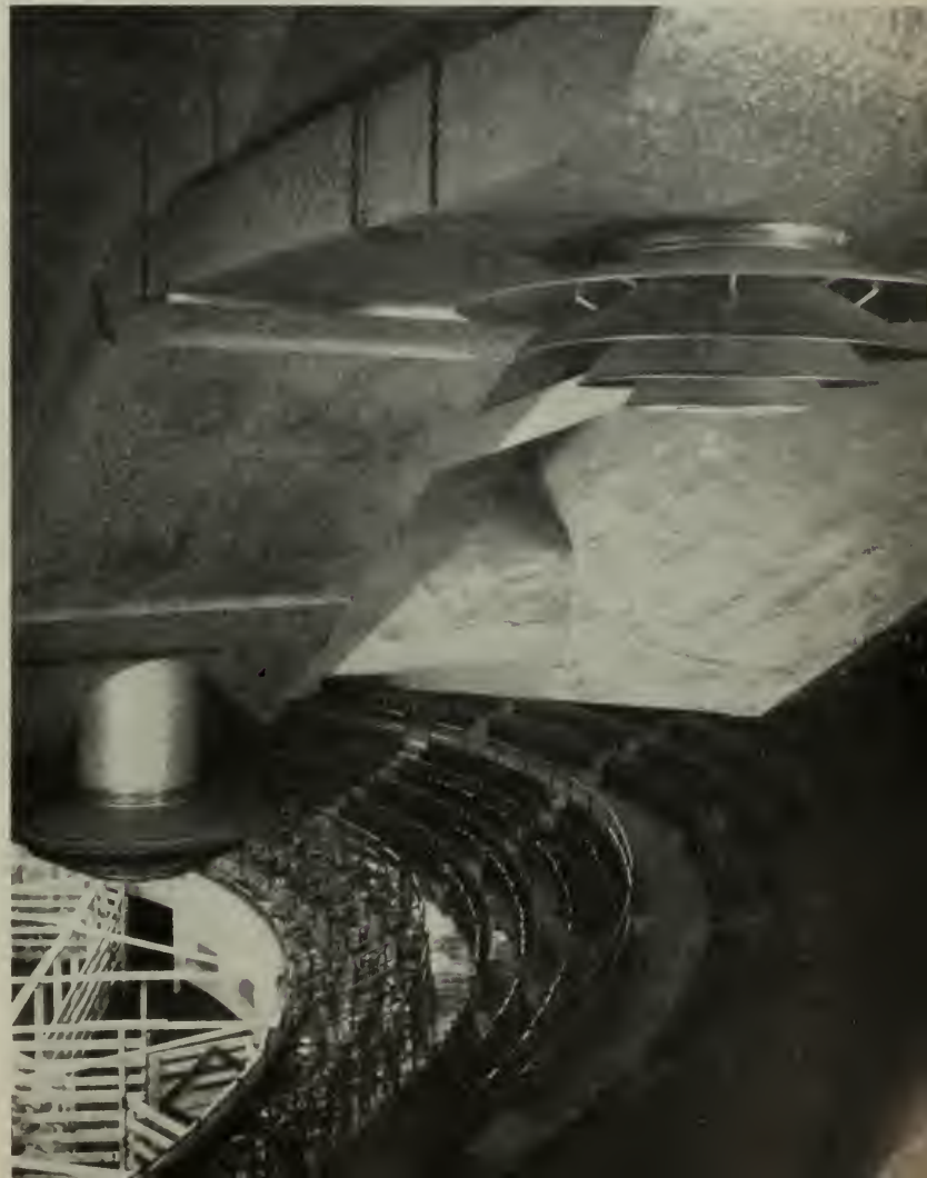
In New York's huge Madison Square Garden, conditioned air is distributed at 400,000 cfm in a manner that supplies 22 cfm to each of the 18,500 spectators without causing drafts. Two of the 102 Anemostat air-diffusers used in this installation are seen here.
