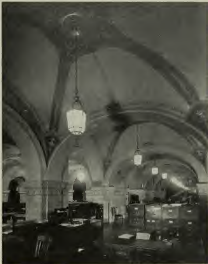
Only scientific air-diffusion could afford proper air-distribution in this room with a vaulted ceiling. Here at the Bank of America, Los Angeles, air enters the room through Anemostats. Lighting fixtures are suspended from each of these air-diffusers.
