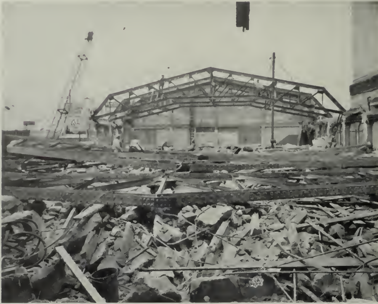
BALCONADE BUILDING comes down. Structural steel supporting roof over ballroom being removed by large crane shown at left.
