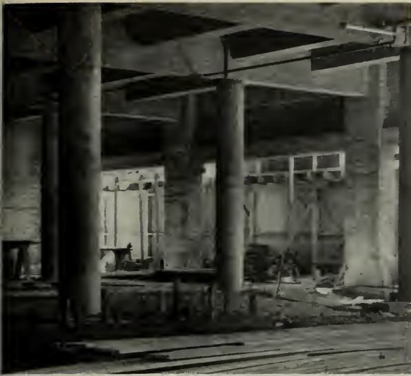
ROUGH INTERIOR: Showing sturdy reinforcing of floors and concrete pillars for upper floor support.
