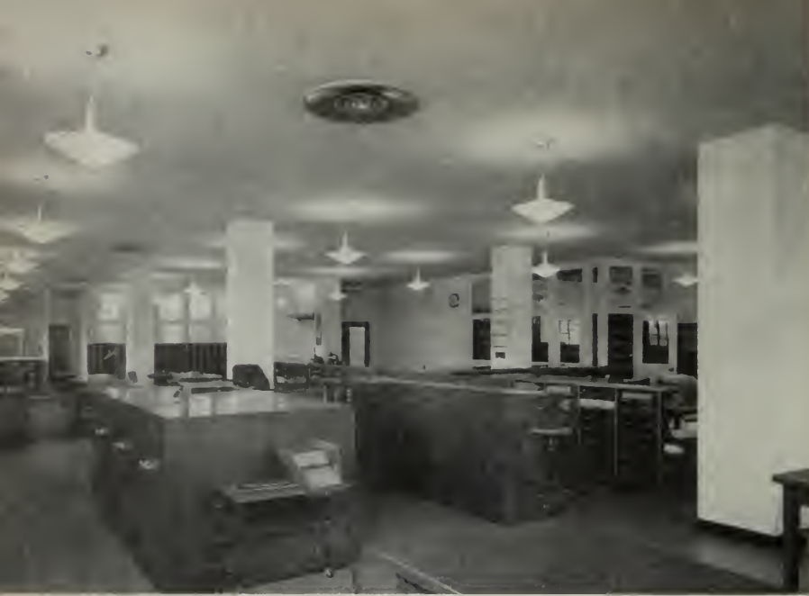
Air-diffusers insure uniform distribution of air throughout virtually all types of public buildings. Here in the Stanislaus County (California) Court House, these devices are seen on the ceiling.
