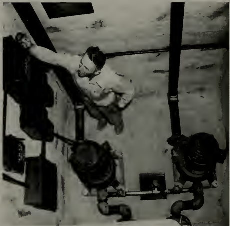
Sump Pit showing pump equipment
