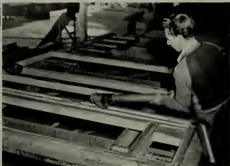
Modern methods of home construction are the result of planning by architects to facilitate erection and to make a better-built and more livable home for post-war living. Here the wall sections in a flat-bed jig are receiving glue applied by workman from a glue gun. Construction with glue not only makes stronger walls, but saves tons of nails which would ordinarily be used.
