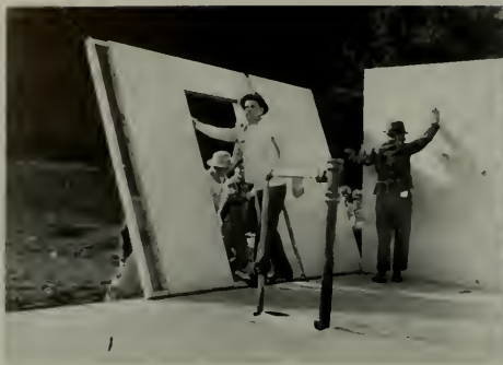
Because every step in the building and erection of this home was planned to the nth degree before a piece of lumber was cut, it goes up as easily as a house of cards. This is one of the houses in a 1000-unit project at Bremerton, Wash., which has been prefabricated in the factory, transported by truck to site, where it is easily erected by workmen in a few hours' time.
