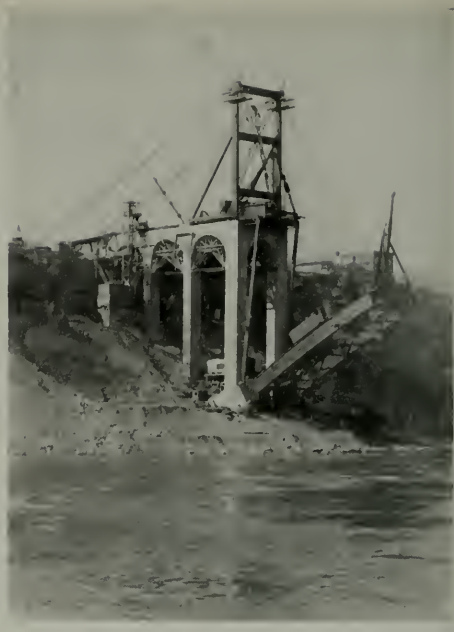
Four sections of arch rib erected with one section cantilevered beyond first tie back. Note: Rib section being moved out to derrick by means of traveler operating on near arch rib.
