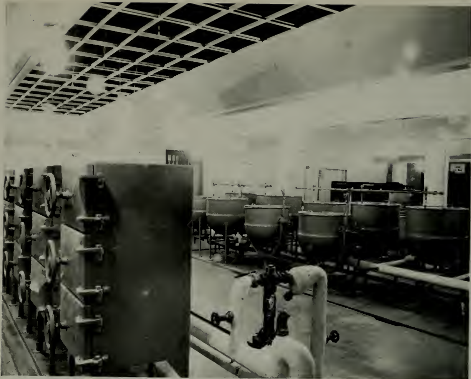
TWO ROWS OF GIANT KETTLES OPERATE LIKE DOUBLE BOILERS, UTILIZING STEAM RATHER THAN BOILING WATER FOR LIQUID COOKING
