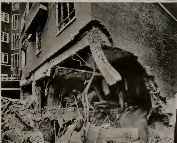
1. Steel-framed structures have the ability to withstand severe punishment from bombing without disintegrating as is the case with plain masonry structures.
