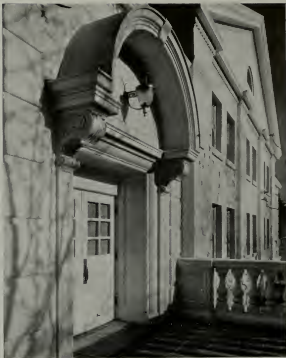
ENTRANCE DETAIL, SUNDAY SCHOOL UNIT, FIRST CHURCH OF CHRIST, SCIENTIST, BEVERLY HILLS, CALIFORNIA
