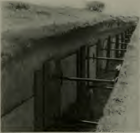
SEWER TRENCHES SHEETED WITH PLYWOOD PANELS. INSTEAD OF THE CUSTOMARY SUPPORT OF TIMBER SHEETING. STANDARD 4 x 8 FT. CONCRETE FORM PANELS OF 3/4 IN. DOUGLAS FIR PLYWOOD.
