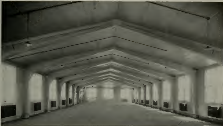
THREE YEAR OLD STRUCTURE AT MADISON, WISCONSIN, FOR U. S. GOVERNMENT PRODUCTS LABORATORY. NOTE WALLS, CEILING AND WEBS OF BUILT-UP LAMINATED ARCHES.
