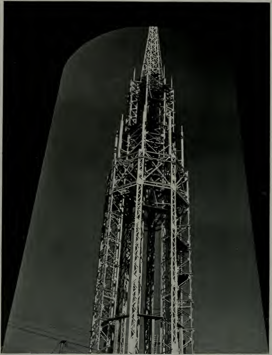
STRUCTURAL STEEL FRAMING OF CENTRAL THEME TOWER, GOLDEN GATE INTERNATIONAL EXPOSITION, TREASURE ISLAND
