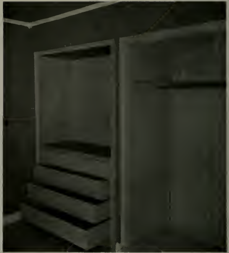
CONSTRUCTION PICTURE DURING REMODELING OF THE HARRISON CLARK HOUSE. DOUGLAS FIR PLYWOOD USED FOR CLOSET AND BUILT-INS.
