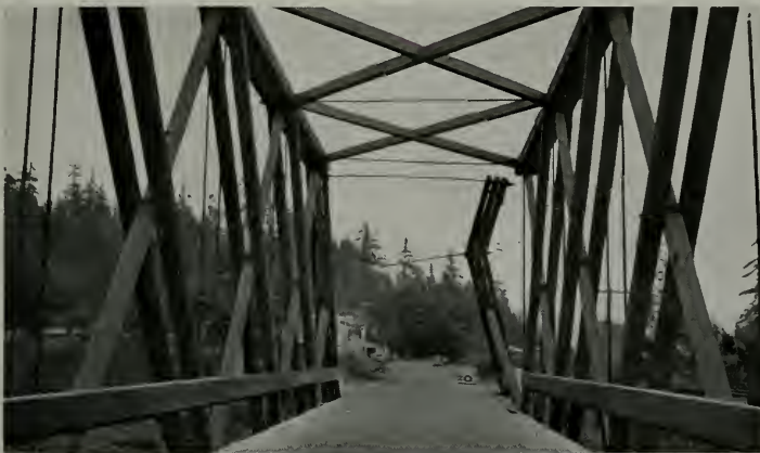
YAGER CREEK BRIDGE IN HUMBOLDT COUNTY, CALIFORNIA. NOTE BROKEN END POST.
