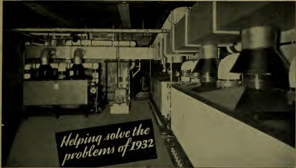
The two automatic gas-fired steam boilers, at right, furnish efficient service to approximately 8,000 square feet of cast iron radiation. The third automatic gas-fired boiler, at left, is connected to two 2,000-gallon tanks, equipped with steam coils for hot water supply.
