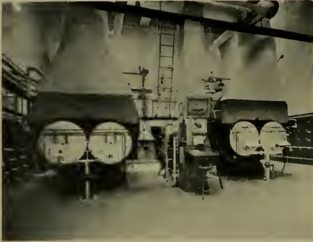
BOILER PLANT, SOUTHERN PACIFIC BUILDING, SAN FRANCISCO
