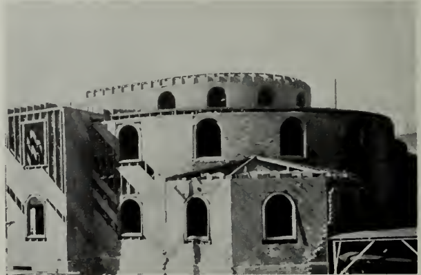
BRICK VENEER CHURCH, SACRAMENTO, IN PROCESS OF DEMOLITION, SHOWING WOOD FRAME IN PERFECT CONDITION
