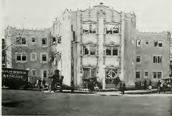
Showing Interlocking Tile Walls of Bennett Apartment House after fire Not a tile cracked—not even a crack in the stucco
