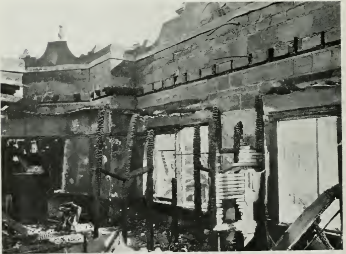
BENNETT APARTMENT HOUSE, STOCKTON Note splendid condition of hollow tile walls after exposure to flames
