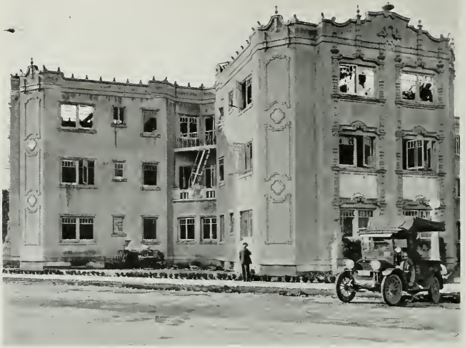
BENNETT APARTMENT HOUSE, STOCKTON Showing condition of hollow tile walls after fire
