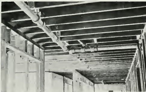
CORROSION DRAIN LINE IN VOCATIONAL HIGH SCHOOL, OAKLAND
