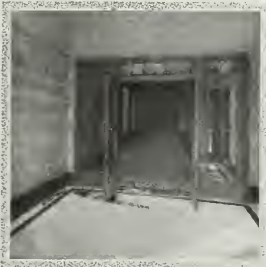
In the vestibule entrance, as well as in the elevator hall, Batesville Marble has been used as the floor material. The walls are Napoleon Gray, ceiling high, with a floor border and base of Blue Belge. Italian American Marble Co., Contractors.
