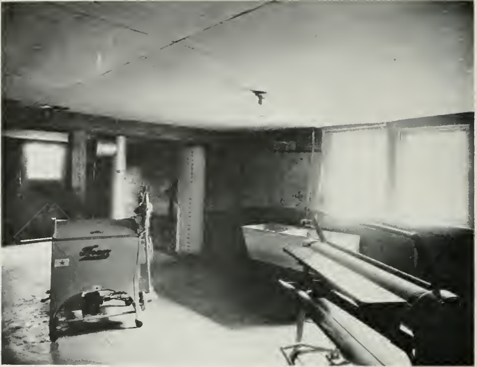
LAUNDRY, COMPLETE ELECTRICAL HOME, SAN FRANCISCO Equipped with Thor electric washing machine, ironer and electric water heater
