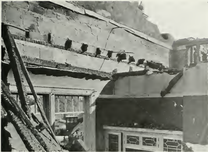
BENNETT APARTMENT HOUSE, STOCKTON Roof and partitions destroyed. Hollow tile walls intact
