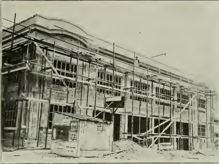
FLIMSILY CONSTRUCTED SCAFFOLD WITHOUT RAILINGS OR TOEBOARDS.
