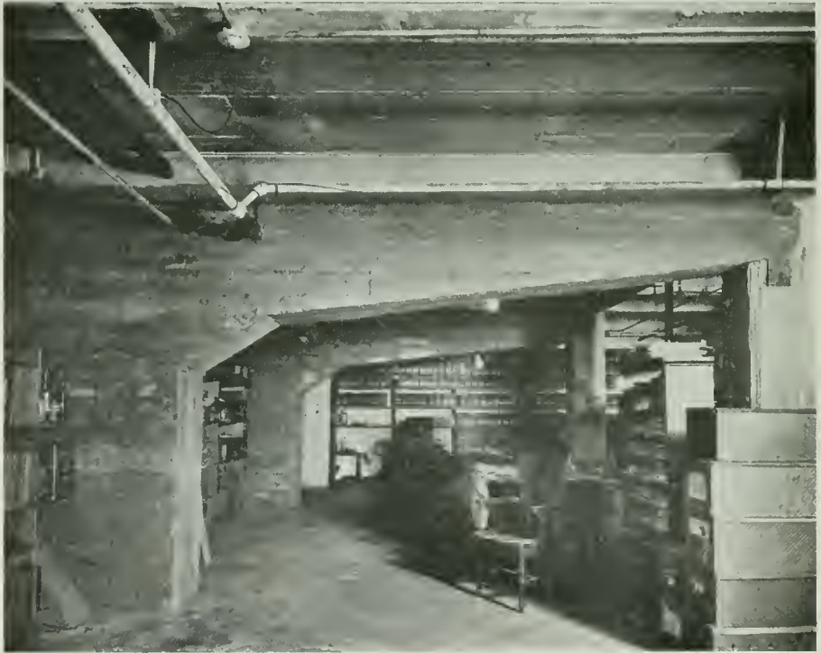
CANTILEVER IN BASEMENT AT INNER PROPERTY LINE COLUMNS, ROBERT DOLLAR BUILDING, SAN FRANCISCO CHAS. W. McCALL, ARCHITECT
