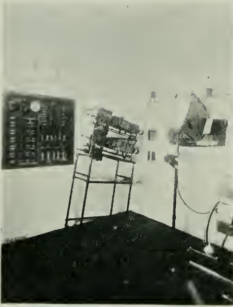
Operating Room, Showing Dissolver Control
