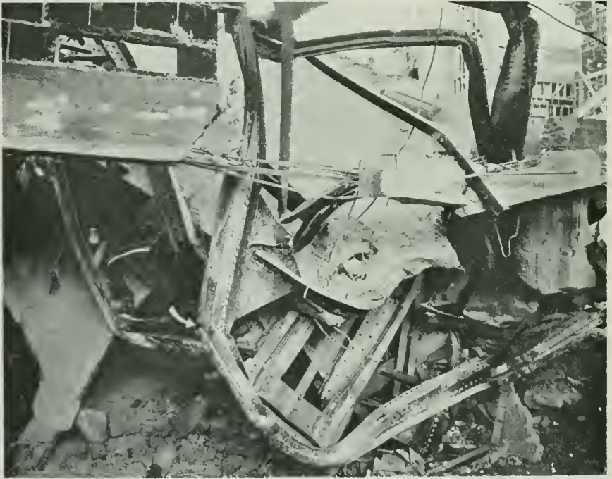
ARROW POINTS TO BREAK IN BOTTOM CHORD OF TRUSS D, REFERRED TO IN TEXT
