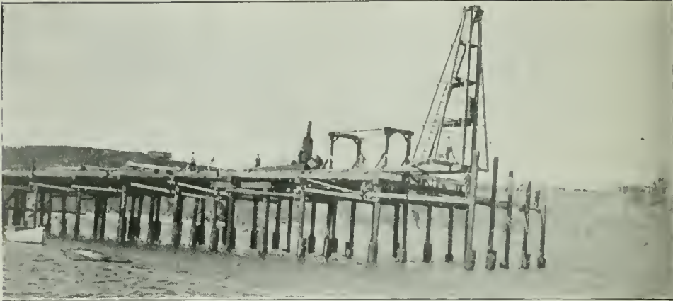
Fig. 1—This photograph shows the use of Armco ingot iron corrugated pipes to protect a wharf, recently built at Port Orford, Curry County, Oregon, from the ravages of the teredo.
