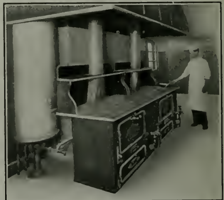
Crude Oil Burners Operating Kitchen Ranges in Government Barracks at Fort Winfield Scott
