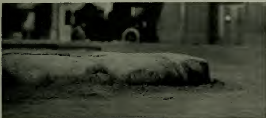
SPALLING OF GRANITE CURBING FROM TRAFFIC
