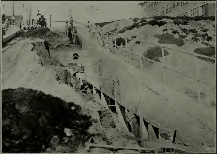
DESTRUCTION OF STORM DRAIN AT LONG BEACH, CALIFORNIA
