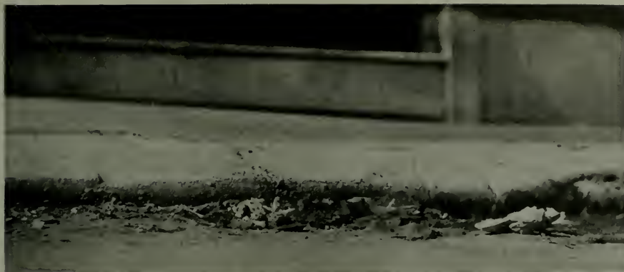
RESULT OF ABRASION ON GRANITE CURBS
