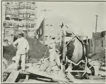
Foote Batch Mixer with Power Loading Skip, on building construction Lange & Bergstrom, Contractors.
