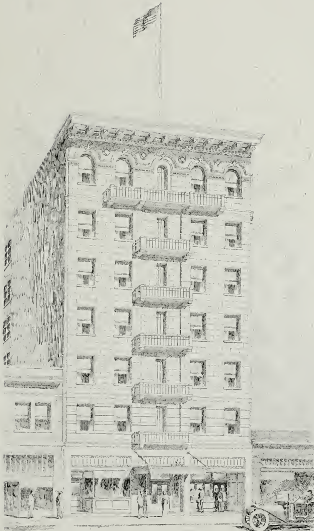
Hotel for Joseph Wagner Now Under Construction, San Francisco T. Peterson Ross, Architect. A. W. Burgren, Engineer Plumbing Fixtures by the R. W. Kinney Co.
