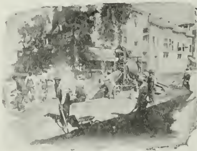
No. 6A Mixer with Gravity Distributing Chute on paving work at Chico, California. Ransome-Crummey Co., Oakland, Cal., Contractors.
