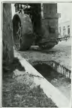
Part circle, with 30-inch base and 14-inch rise at center, made of 14 gauge iron, supporting 14-ton roller. Culvert installed in city of San Bernardino.
