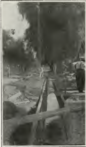
Part circle Culvert, 16 gauge, 14-inch base by 7-inch rise, 68 feet long, with two tees 17 feet long, at Sixth and Lime streets, city of Riverside
