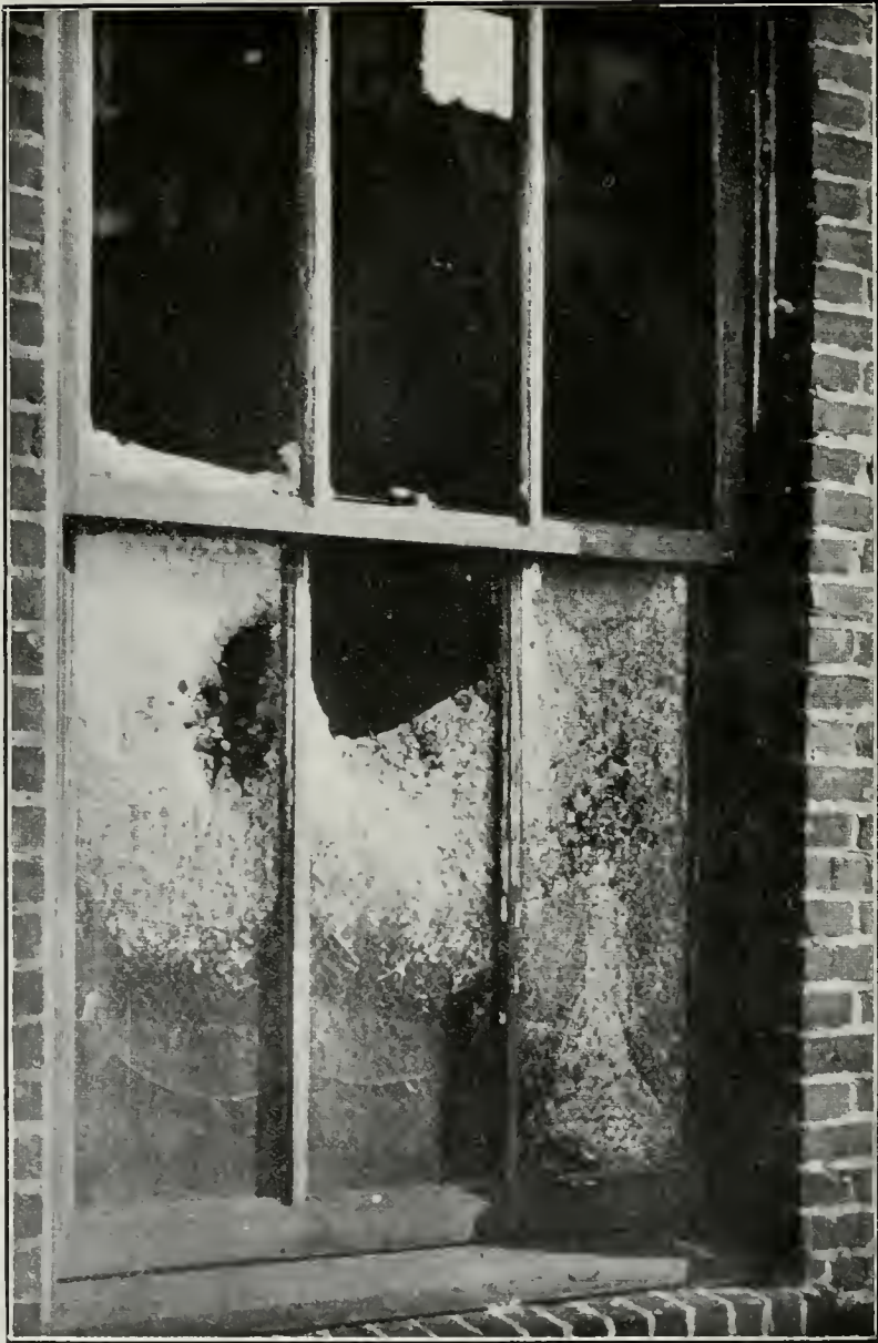
Failure of Wire Glass from Exposure by Fire Within a Building. Note Satisfactory Condition of Metal Frames, and that Glass Alone Failed
