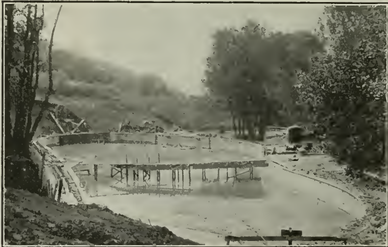
CONCRETE SWIMMING TANK, UNIVERSITY OF CALIFORNIA, BERKELEY, CAL. WATERPROOFED WITH MEDUSA COMPOUND
