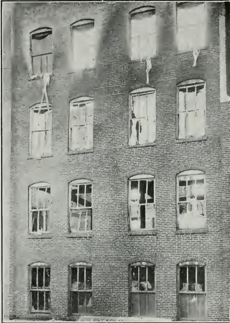
Another View Showing Effect of Exposure of Wire Glass Windows from Fire Inside Building
