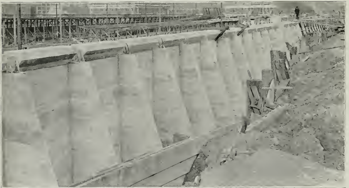
Rear View of Fifth Avenue Retaining Wall, O.W. R. R. & N. Co. Terminal, Seattle
