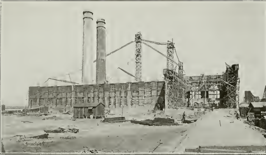
Progress Work on the Edison Plant, Redondo Contractor, F. O. Engstrom Company
