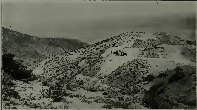
II. Los Angeles Aqueduct—Preliminary Road Construction and Power Line, Grey Ridge, Jawbone Section
