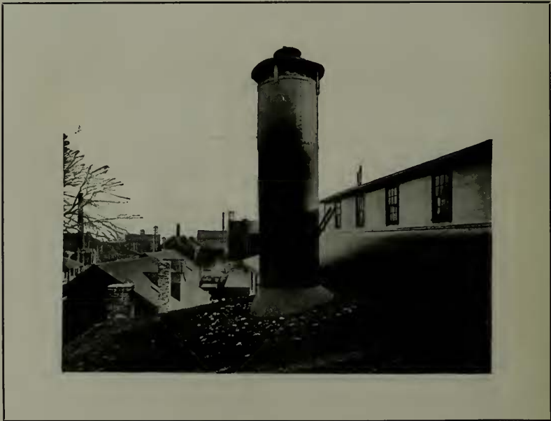
Cupola Stack of Woburn Machine Company, Woburn, Mass., demonstrating durability and fire-proof qualities of Asbestos Protected Metal
