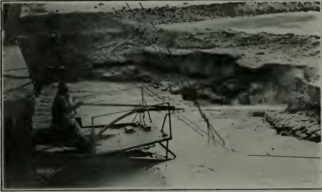
III. Los Angeles Aqueduct—Hydraulic Dredge Under-Cutting Face of Bank With Stream of Water Under High Pressure
