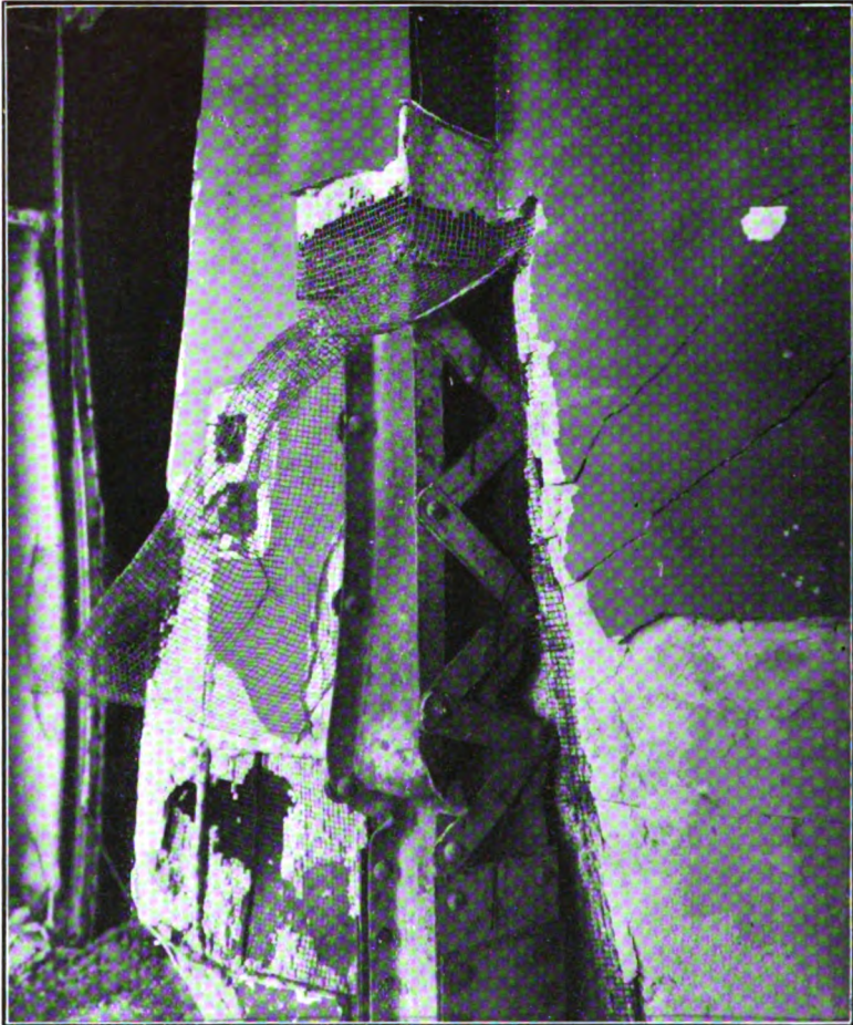
Buckled Column in the Hotel Alexander, San Francisco
