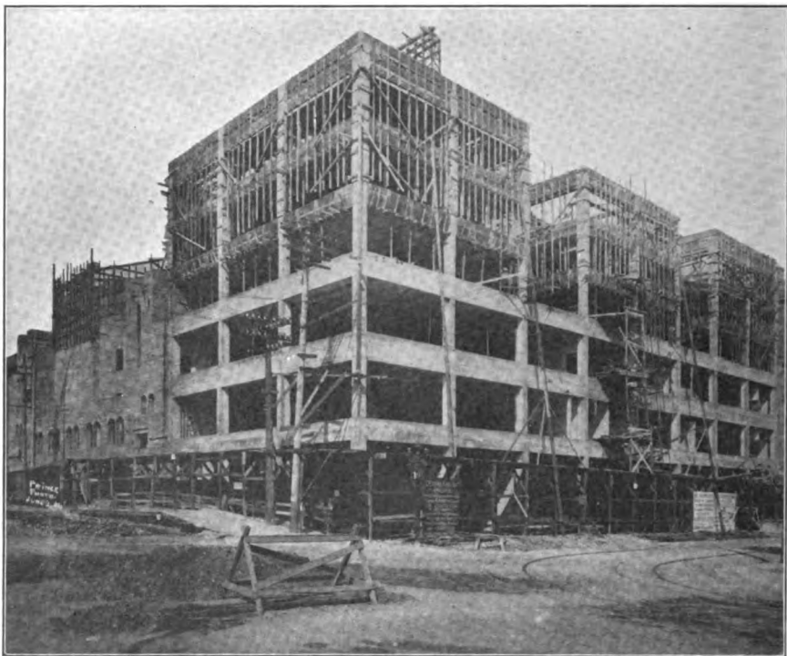
Progress Work on Reinforced Concrete Auditorium. Los Angeles. Showing Office Portion of Building Chas. F. Whittlesey, Architect
