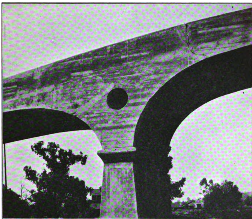
North Face East End of Big Arch. Reinforced Concrete Bridge, South Pasadena Showing Crack on the Right
