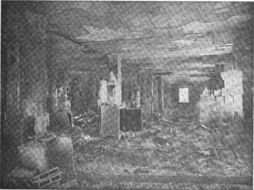
Effects of the Heat on the Fire-proof Tiling in the Union Trust Building
