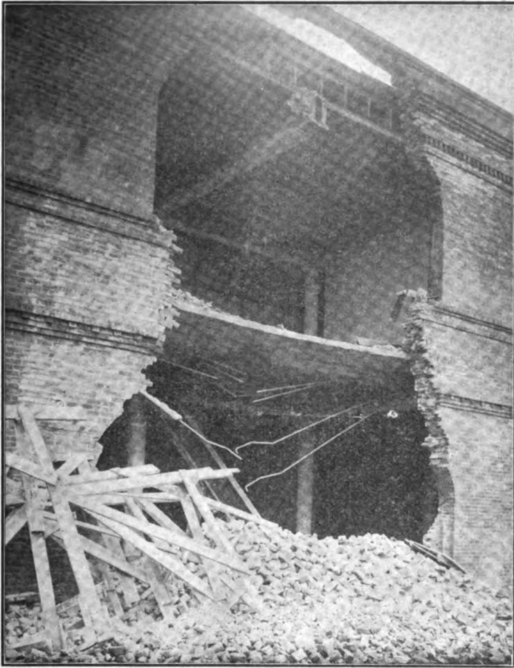
Fig. 4. The Casa Calwa Building, Townsend Street Near Third, Showing How the Reinforced Concrete Floors Remained in Position After the Supporting Walls Had Been Demolished by Explosions in the Adjoining Building Meyer & O'Brien, Architects
