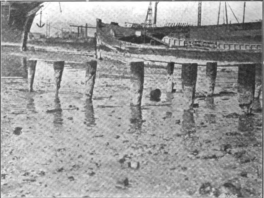
Wooden Piles and the Hull of a Wooden Vessel, Showing the Destruction Wrought by the Teredo and Limnoria From a Photograph Taken April 17
