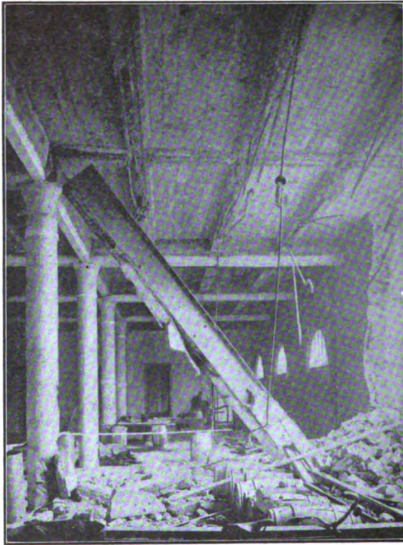
Fig. 5. Interior View of the First Floor of the Casa Calwa Building Meyer & O'Brien, Architects
