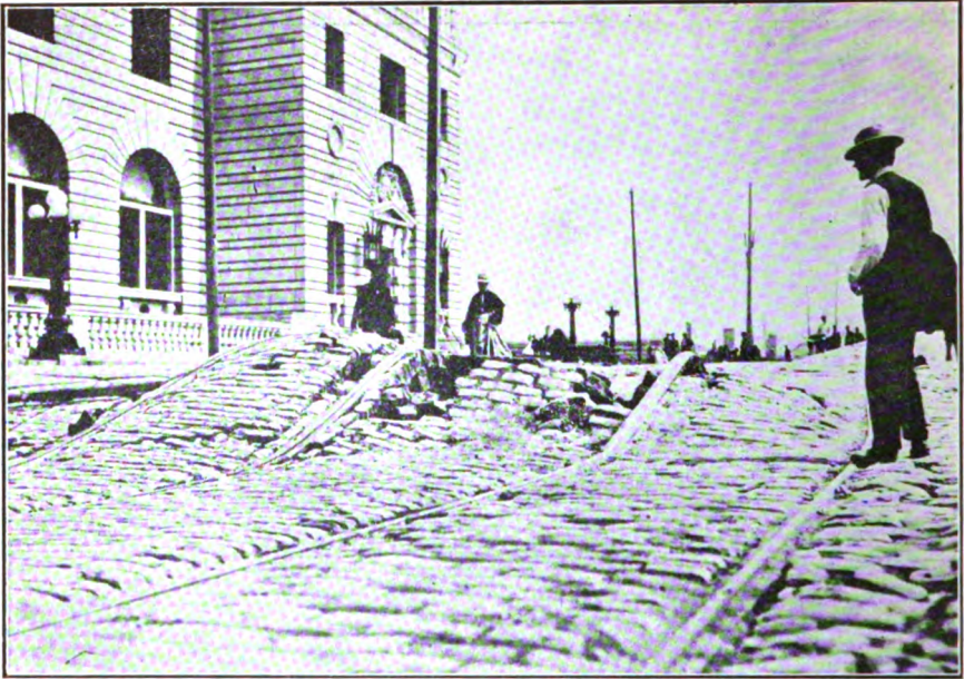
Postoffice Building, San Francisco, Showing Effect of the Earthquake on "Made" Ground in Front of the Building.
