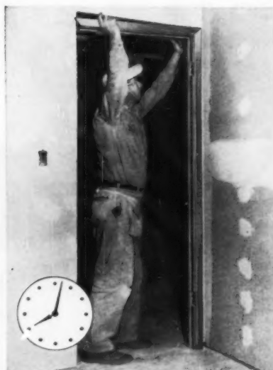
8:02 a.m. Place header in starting position and rotate to horizontal position. Note trim hairline-mitered corner. Provides neat, professionally-finished appearance without on-the-job fitting.
