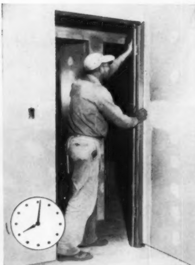
8:01 a.m. Hinge jamb is placed in starting position and rotated to vertical. Lightweight sturdy 22 gauge, rust-resistant steel sections are easy for one man to handle.
