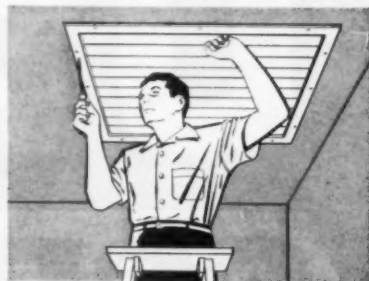
Step 3 Screw-fasten automatic ceiling shutter. Metal trim covers edges of opening. No finishing necessary.
