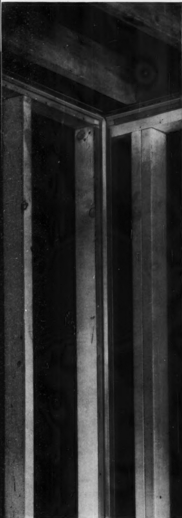
First step in the "Steeffast" system is placing the steel member in corner and ceiling joints.
