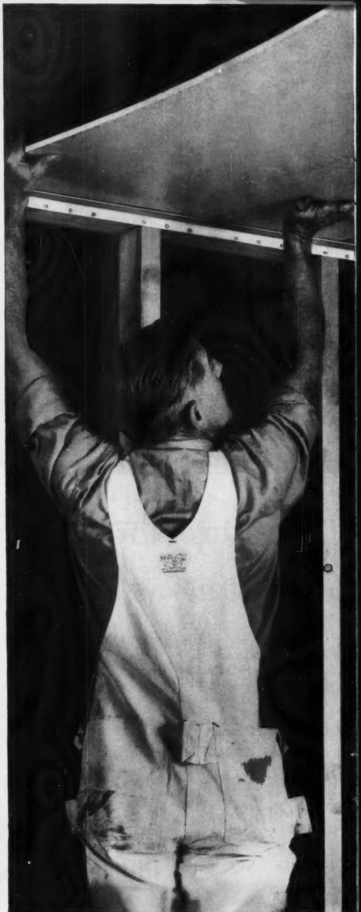
The center ceiling panel is bowed slightly and slipped into the ends of the "Steeffast" member.
