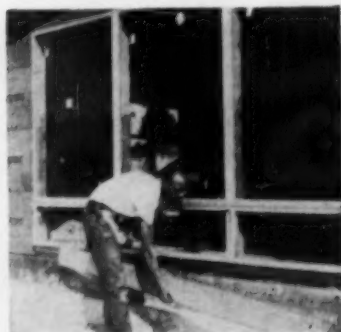
SIX: After windows are in and mullioned to awning frames, temporary board is removed. (Elapsed time: 20 min.)
