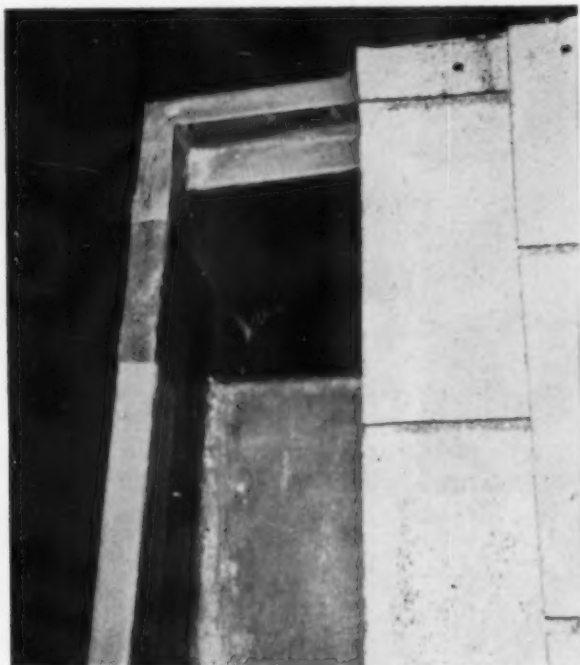
DRAIN OPENING is placed at lower end of roof. Although no downspout has been attached, conventional type can be used. Variation of this is a concealed downspout, led back through roof overhang and down to the drain via interior wall of the home.
