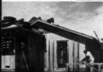
Rowland Van Ness used Exterior Fir plywood and batten siding to eliminate all sheathing, bracing and blocking.
