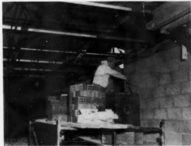
OPEN WEB bar joists of steel support upper-level flooring. Front half of nine-room house is built on slab, back half is over a basement.
