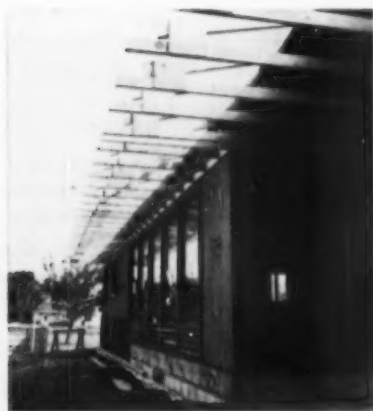
ROOF JOIST ends are prepared to receive wooden gutter. Notched area takes gutter which is then lined with plastic sheet. The builder fitted the liner at the job site, using sharp knife.
