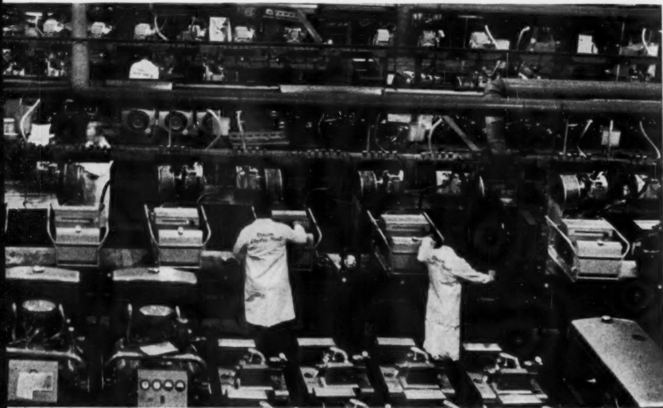
Part of Onan's testing facilities—largest electric generating plant testing area in the industry!
