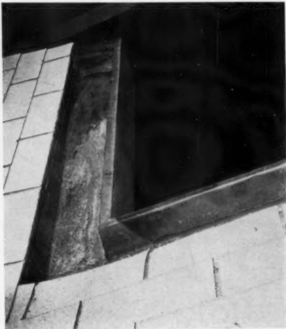
RECTANGULAR WOODEN GUTTER is shown in place at the eave. Note how gutter is pitched to drain by following photo from lower right-hand section to upper left. Saraloy 400 flashing is extended into gutter, contoured with heat lamp or hot air gun. It lines gutter and seals joint between gutter and roof.
