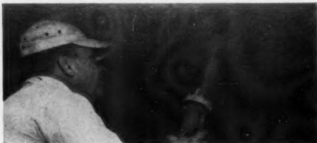
THE DRY ASBESTOS FIBER is ejected from the nozzle of a high-pressure hose where it is air-mixed with water from the nozzle head.
