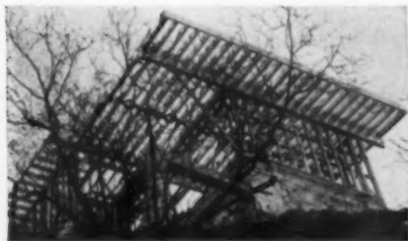
Home designed by Columbia Art Directors Ross Bellah and Carl Anderson; engineered by Victor Gruen Associates, Architects, Beverly Hills and New York City.
