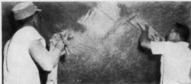
GUN OPERATOR at left sprays 2½" of limpet asbestos material onto bare concrete roof while helper floats and finishes a sprayed area.
