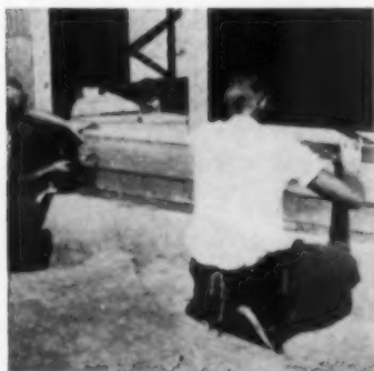
ONE: Temporary board is leveled, nailed along pre-scribed mark. Board supports "Wood-A-Lume" window.
