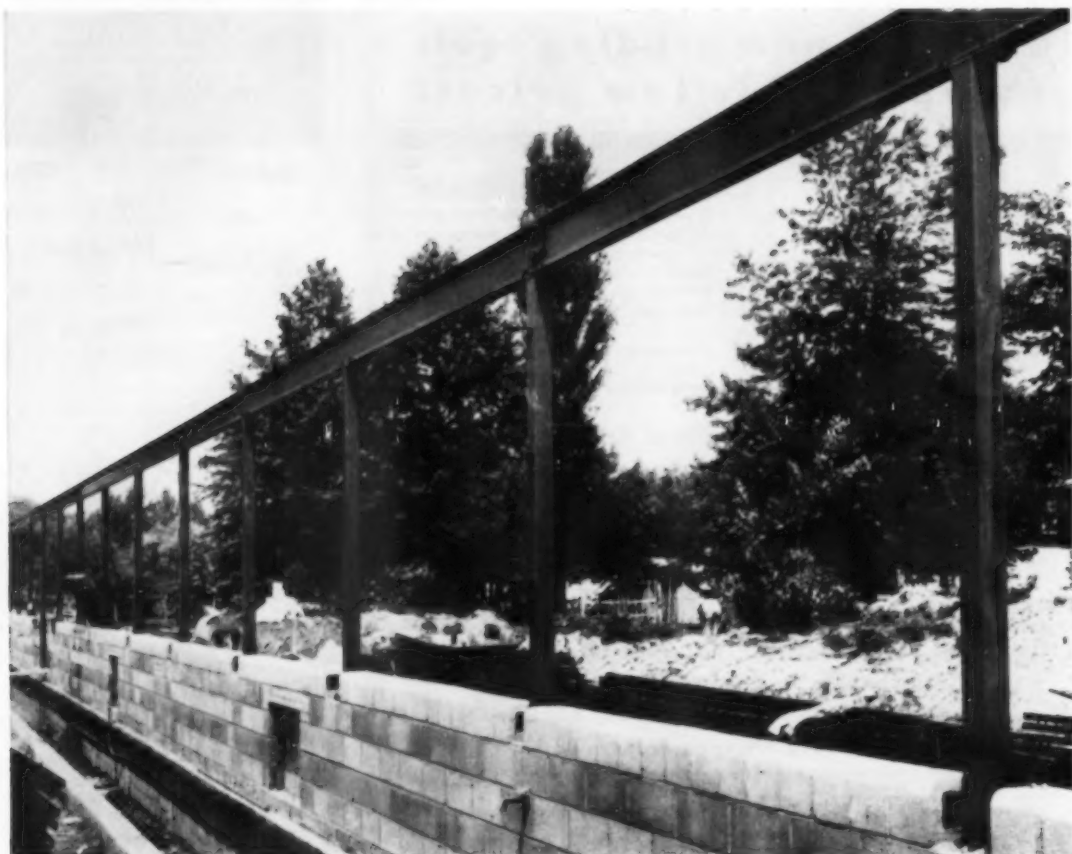
REPUBLIC STEEL 4 x 4" square tubes form framework of elementary school, act as columns, mullions.
