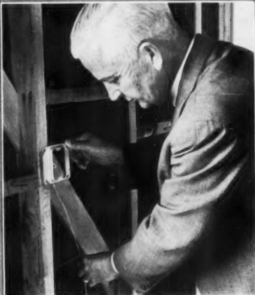
Telephone man Mason Layton checks concealed telephone wiring and position for outlet in a Gardiner "Mission Ranch" home at Fremont, Calif.
