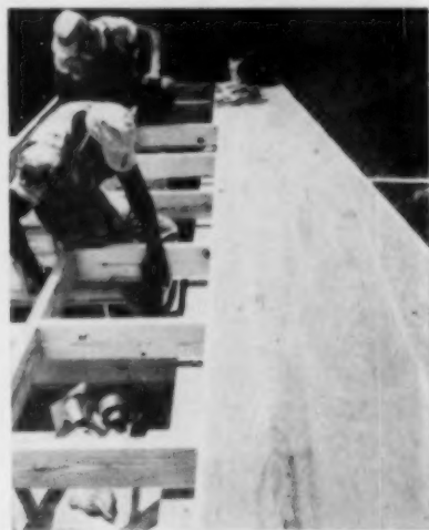
DESIGN AND CONSTRUCTION of "eagle beak" are the same as the standard gable end except for projecting 2x6's.
