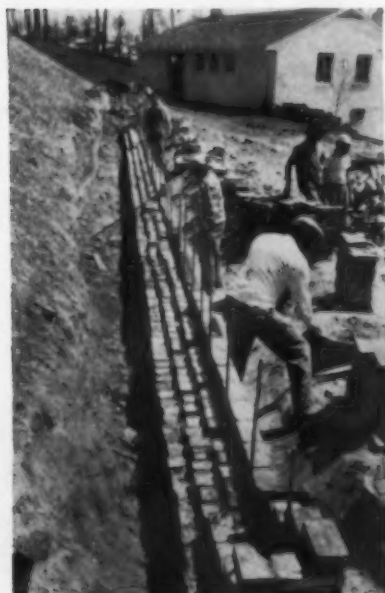
SHALLOW FOUNDATION for wall is dug with trencher. Soil is placed up-hill for later backfilling. Concrete footing is poured, reinforcing set between courses.
