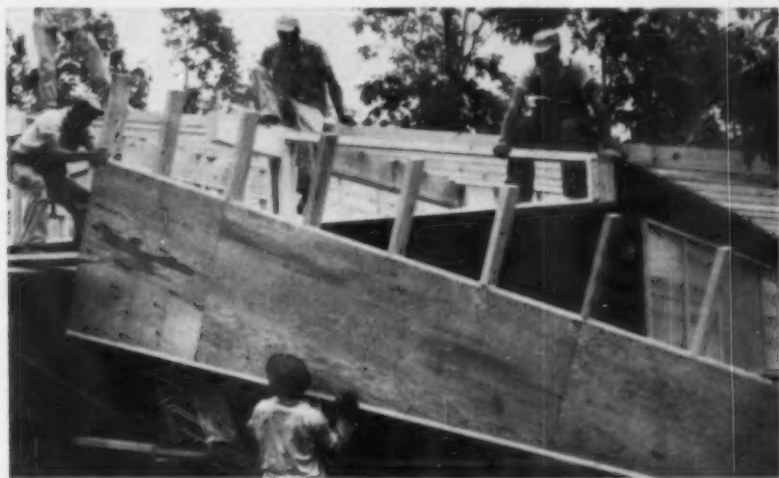
ALTERNATE GABLE RAKE , or "eagle beak," shown above being lifted into position for spiking into first truss beyond the gable. This design is used on more expensive homes than is the straight overhang shown below.
