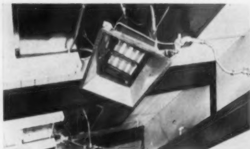
CLOSEUP of overhead Schwank heater, this time at a restaurant in La Puente, Calif. Units are suspended by four chains with a flexible gas connector. A single switch controls their operation. Over-all view, below.
