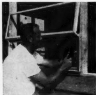
THREE: Center awning window is nailed through its aluminum-and-wood frame, directly into studs.
