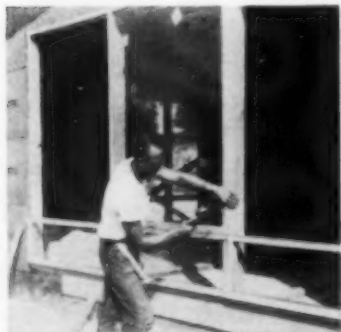
FOUR: The center picture window is nailed in place through prepunched frame, right into the framing studs.
